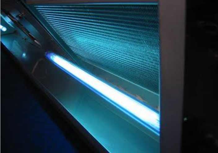
Figure 1 UV Lights in Ducting
